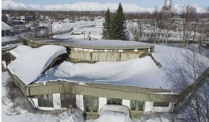
Image 1: Palmer Library Roof Collapse
